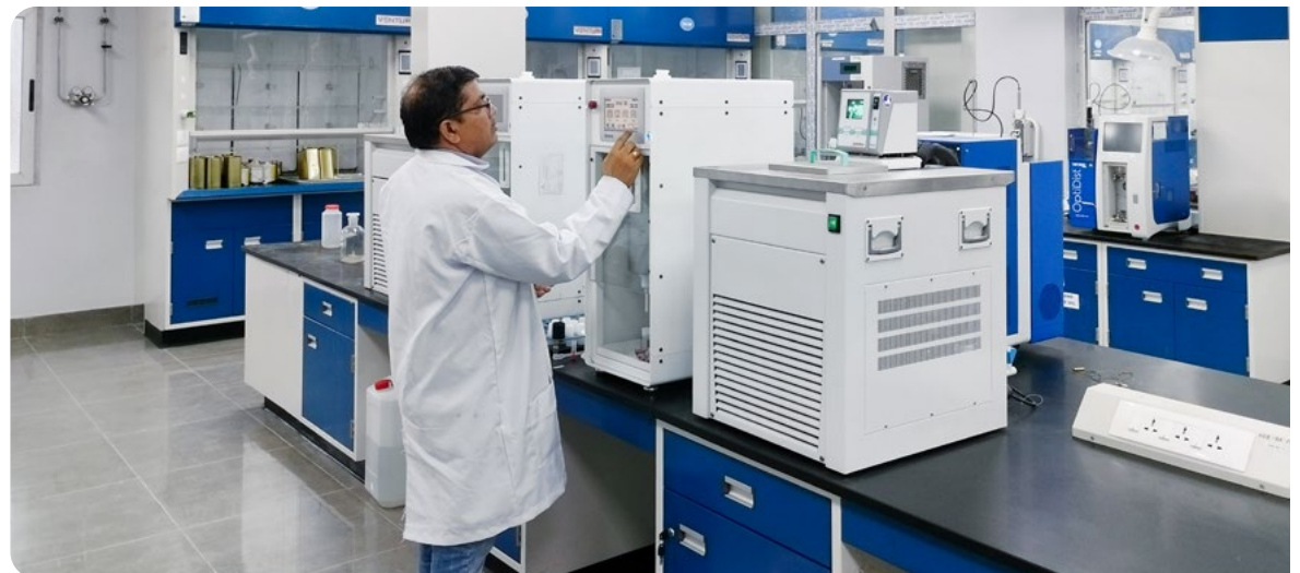
Fixed Steel Casework, Venturi Fume Hoods, Exhaust Systems, HVAC Systems, Gas Distribution
