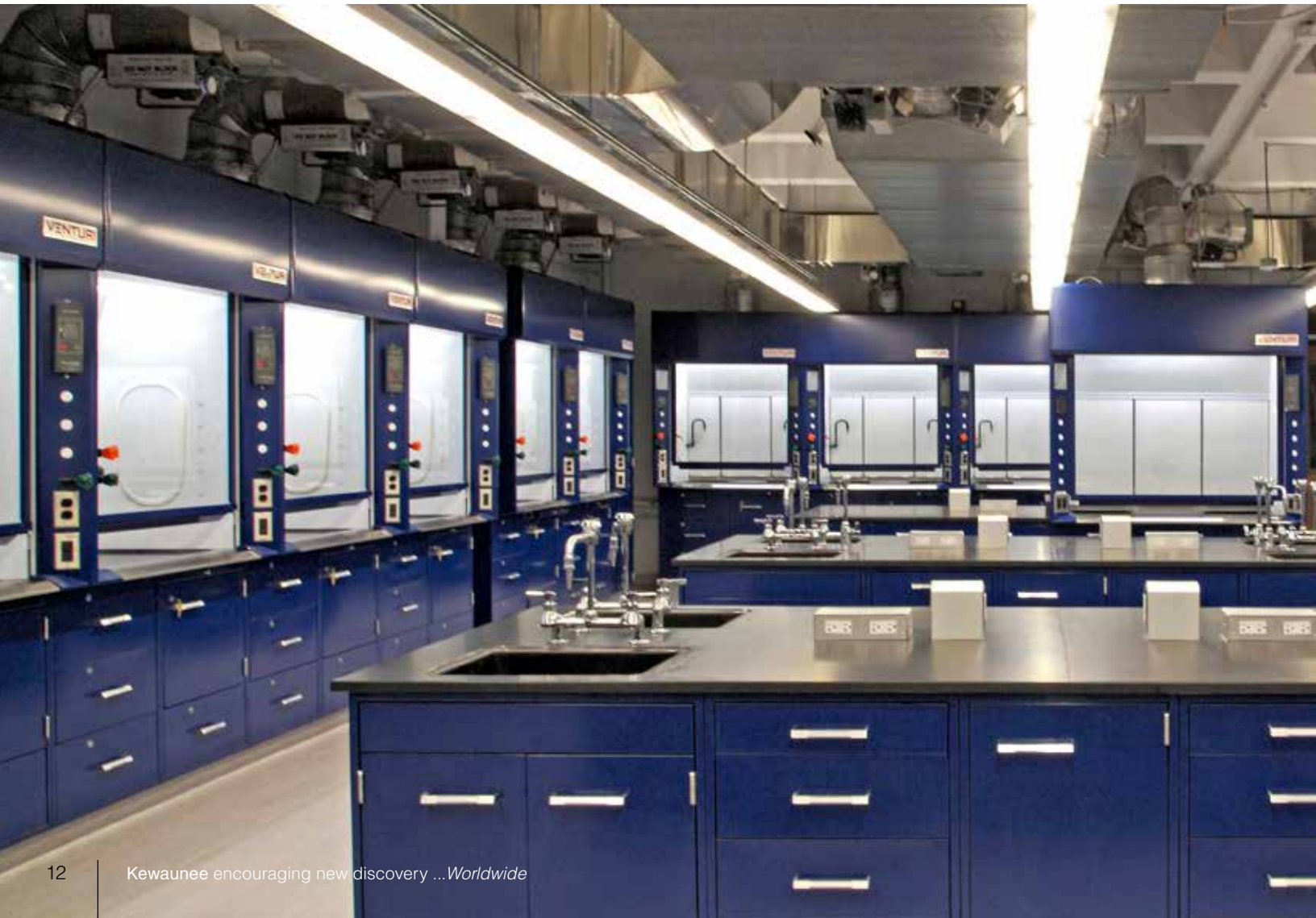
Venturi fume hood lab with multiple configurations
